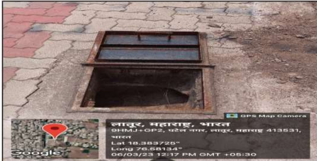
Liquid waste disposal soak pit
