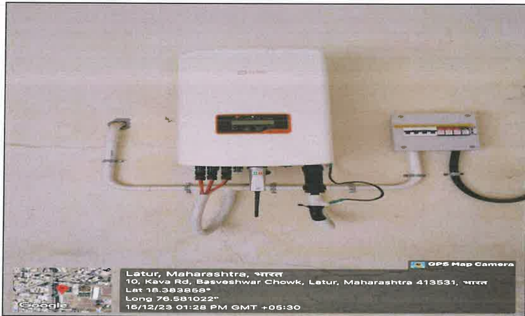
Polycab solar inverter
