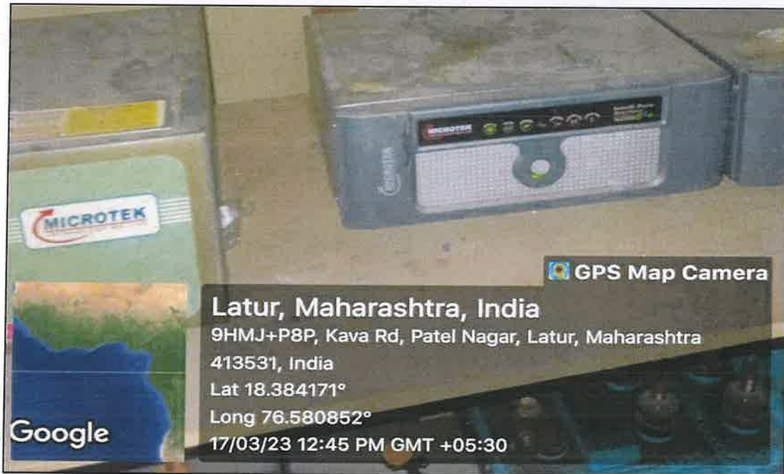
UPS power inverters & Batteries available in college
