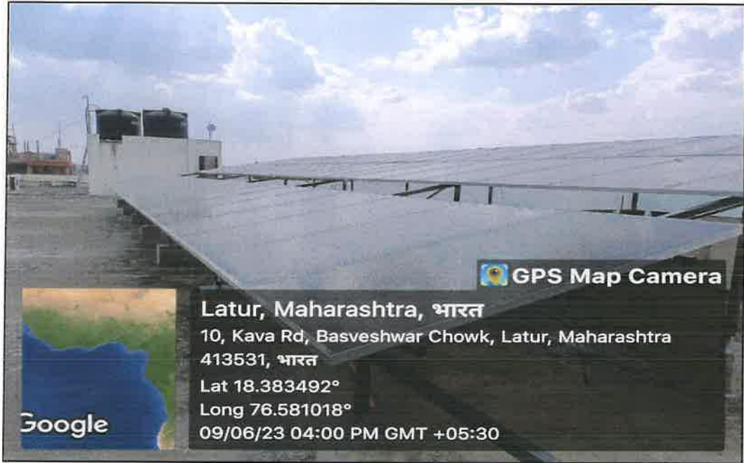
Solar Panel installed at College Rooftop
