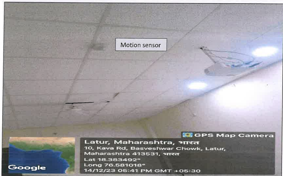
Motion Sensor Lights Installed in Classroom
