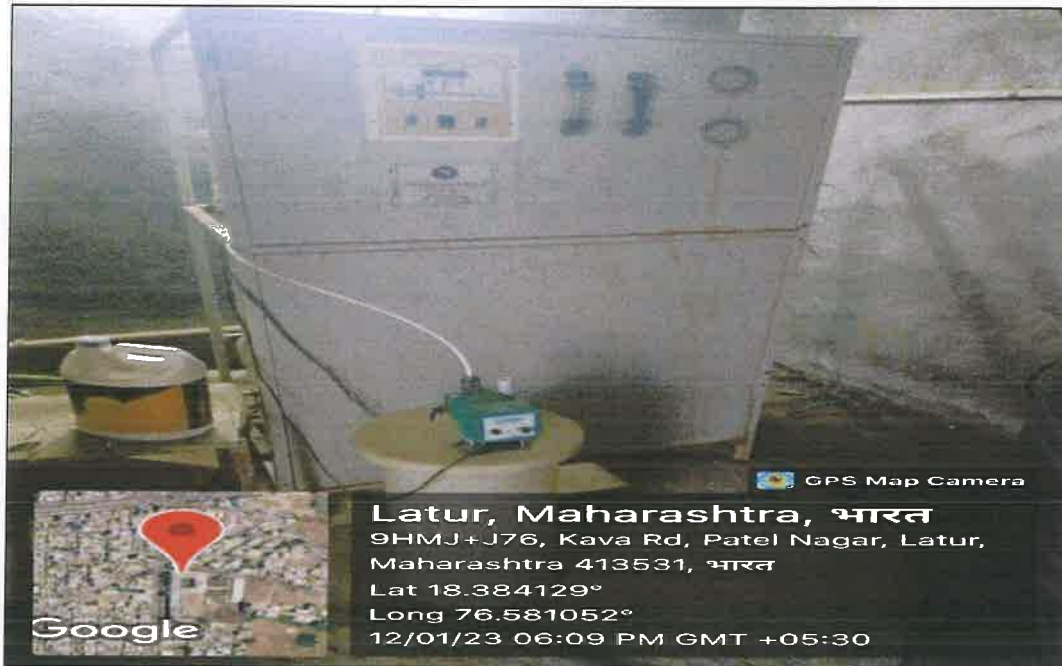
R.O. Water filtration plant
