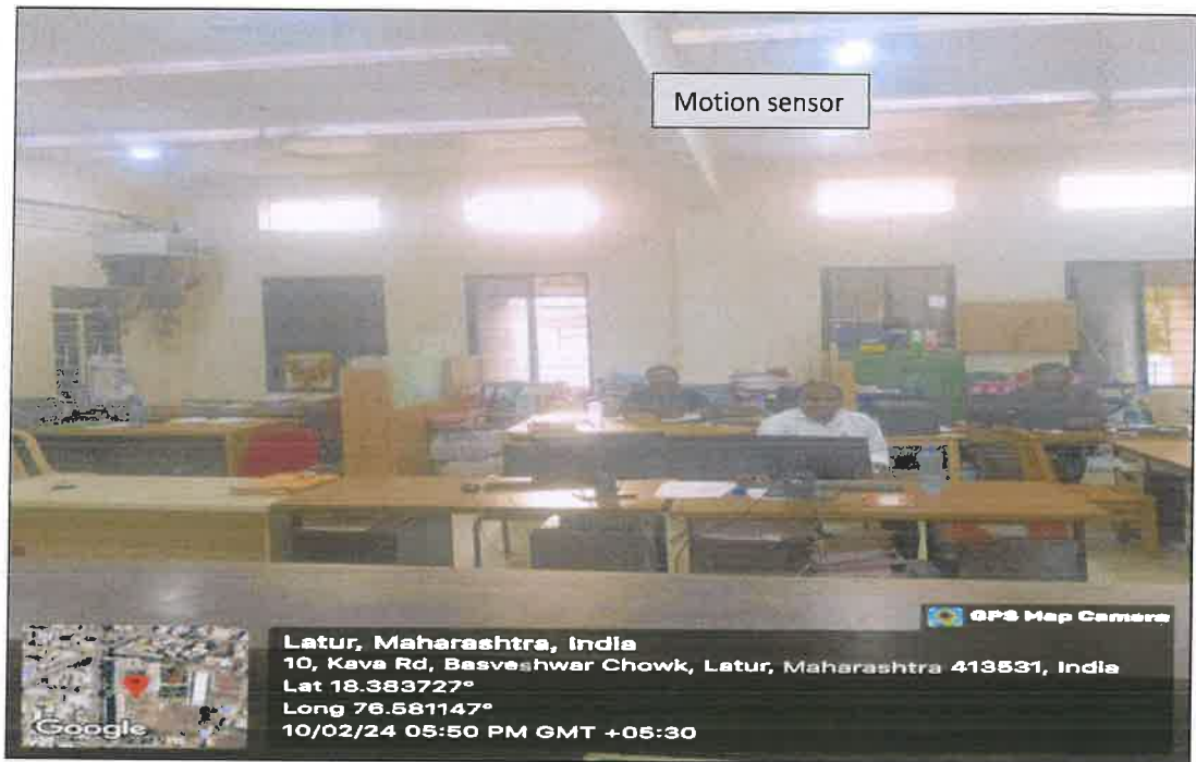
Motion Sensor Lights Installed in administrative Office
