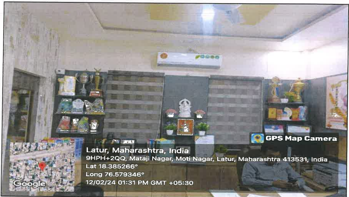
Five Star AC installed in Principal Cabin
