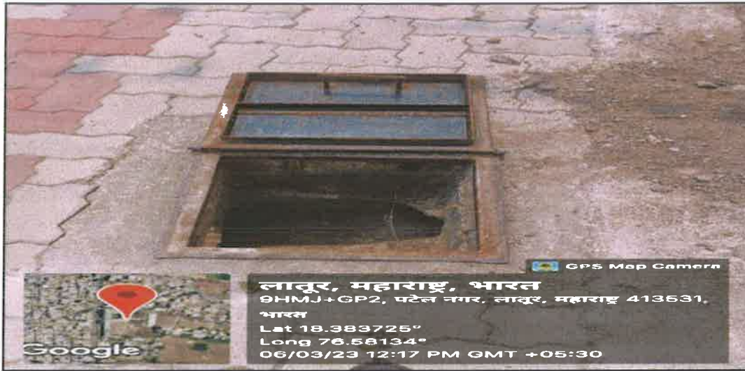
Liquid waste disposal soak pit
