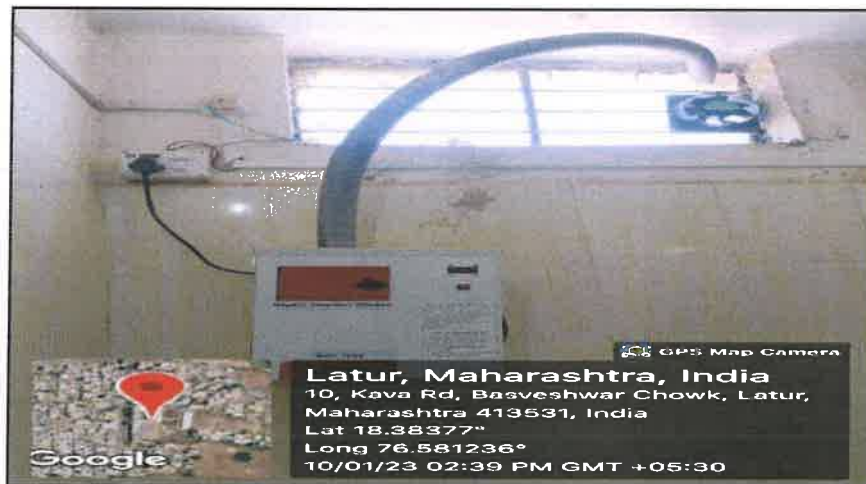
Sanitary Napkin burning incinerator unit
